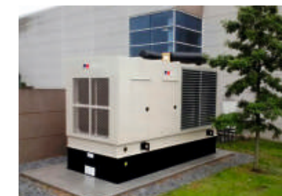
GENERATOR BACKUP FOR LIFT & COMMON AREAS
